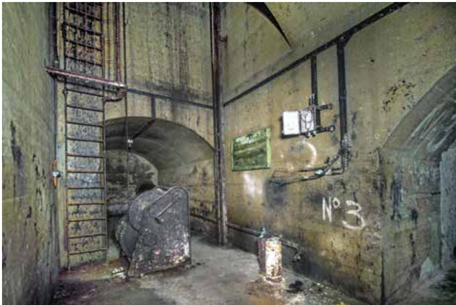
Control chamber for tank No. 3. The 12.2 metre ladder to the upper platform is seen adjacent to the winch. The access tunnel is on the right
